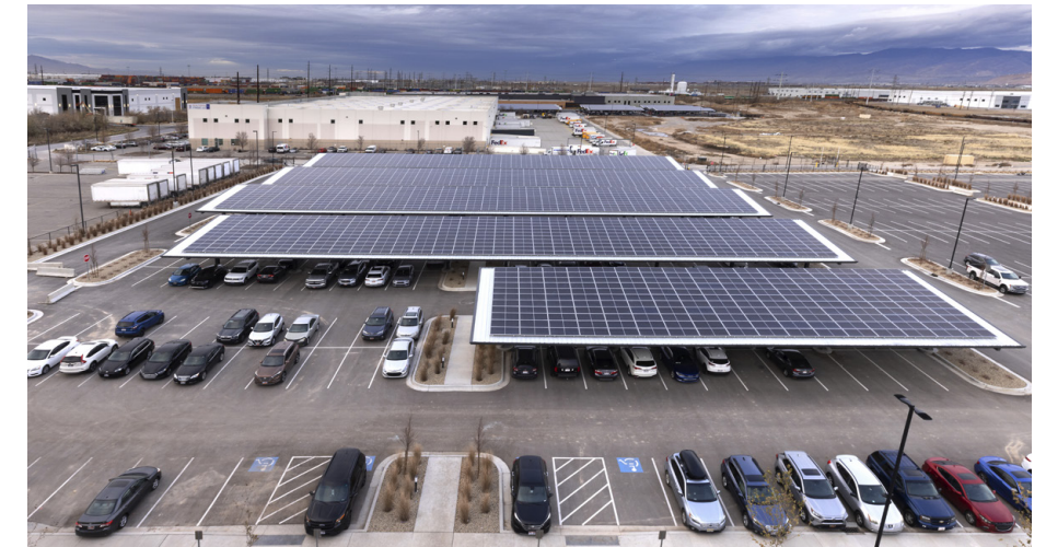
Solar energy is a lever for decarbonization at bioMérieux, like here in Salt Lake City (U.S.).
